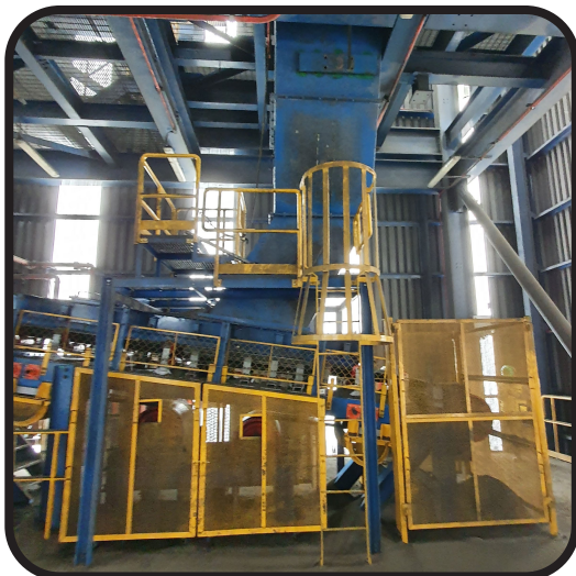
Before Valley Rubber's system was installed
