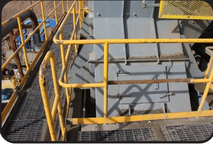
Unsafe access point to the chute
