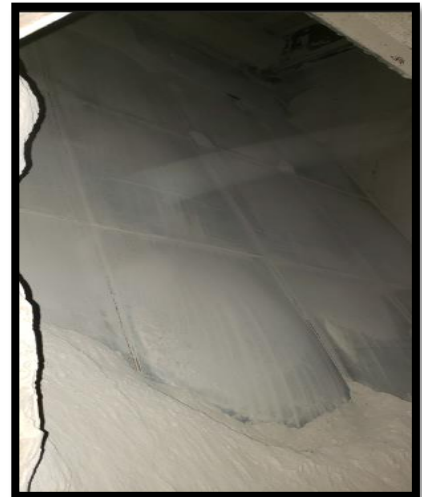
Photos above: Valley Rubber's Inflatable Liners after 1 year in operation without failures.
