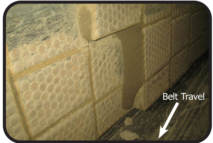
Special geometry is used effectively to relieve the side pressures on the liner package. The liners on the right hand side are inside the Shoe.
