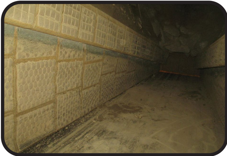
Looking toward the tail of the Loading Shoe. Top left is the engineered ceramic Deadbed Bar that protects the tapered floor of the Shoe.
