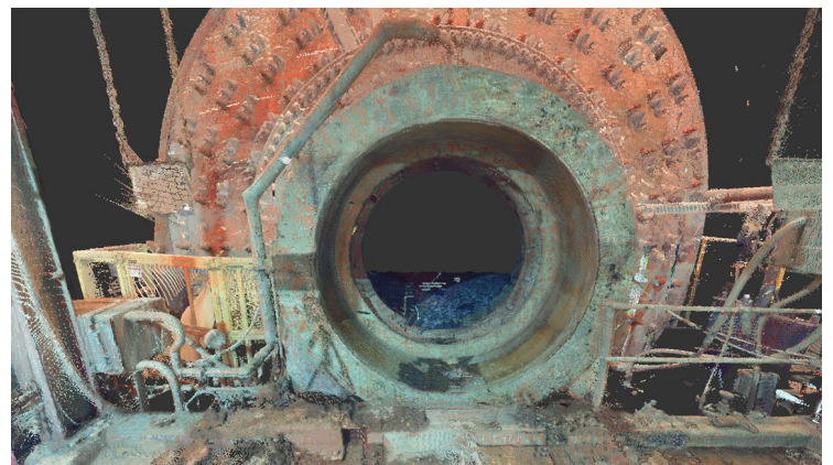
On-site reconnaissance includes: 3D LiDAR scan of your operation, custom Mill Feed Cart design and DEM software to simulate the flow of material.
