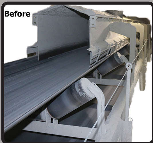
The original design allowed material and dust to escape between the belt and canoe.
