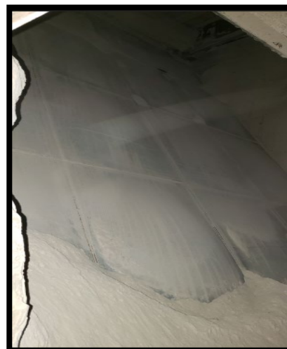
Photos above: Valley Rubber's Inflatable Liners after 1 year in operation without failures.
