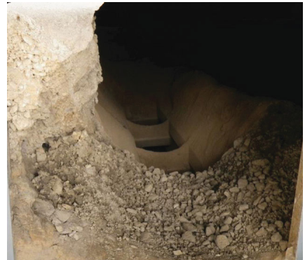
Before: A plugged floor in a screen undersize chute.
