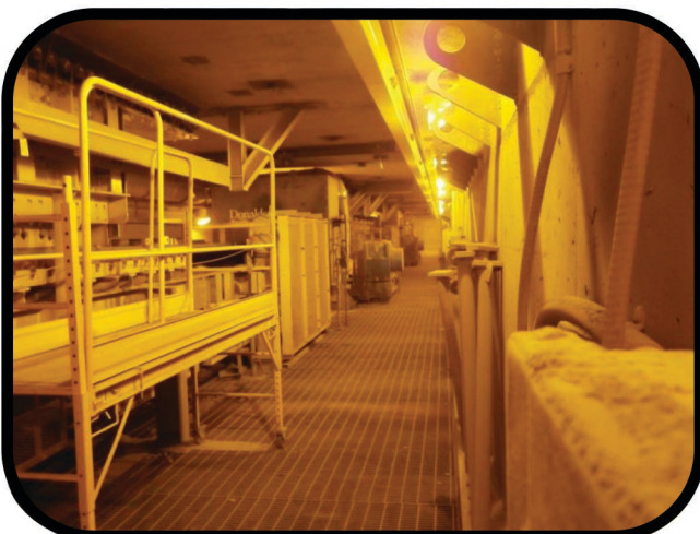
Three 800 TPH Feeders.
