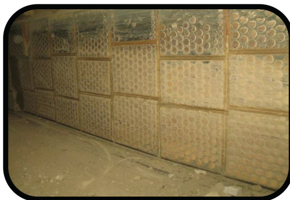
Discharge wall in a 60" feeder
